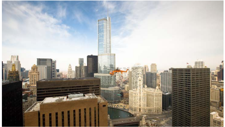
The Hill Group saved thousands of dollars and shortened its project timeline by relying on Erickson Incorporated to place heavy cooling equipment on the roof of a Chicago skyscraper.
