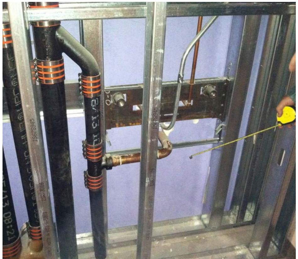
PPM designed—and Jay R. Smith fabricated—a custom lavatory plate that builds in 1/2" of left/right flexibility so PPM can make any adjustments outside the wall, saving a significant amount of time and money. This custom solution is an example of the partnership between the two companies that contributed to successful construction of the new Kaiser Permanente San Diego Regional Medical Center.
