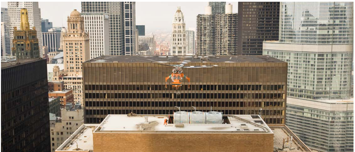
Erickson Incorporated’s Airplane makes short work of rooftop installations, completing two heavy lifts for The Hill Group in less than two hours.
