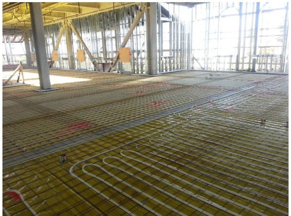
University Mechanical used 75,000 feet of Uponor's 5/8" Wirsbo hePEX™ tubing on three floors on the west side of the building to serve 36,000 square feet of space in the new Aztec Center, one of several energy-efficient features that led to LEED Platinum-certification for San Diego State University's student union.
