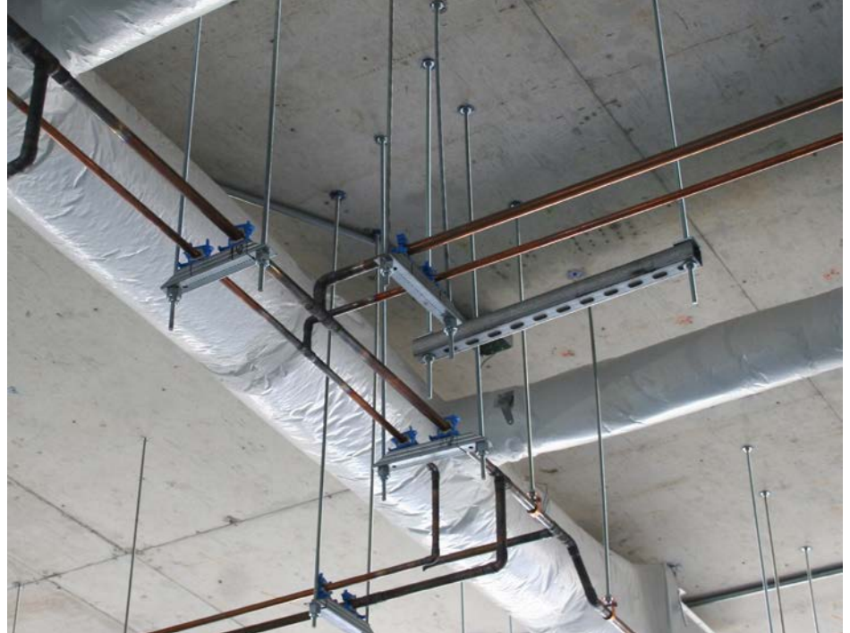
Top: By using CADDY Telescoping Strut Replacement, DSI did not have to cut strut, which saved time and also allowed them to avoid disturbing patients while remodeling a hospital.
